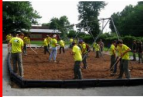
THEY AIN'T PLAYIN' AROUND: Troop #60 builds a swing set for Collins Middle School in West Virginia. This was the most tasking and rewarding community service the group has completed.
